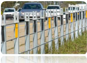
Courtesy of MDOT, the above photo shows a cable barrier system.
