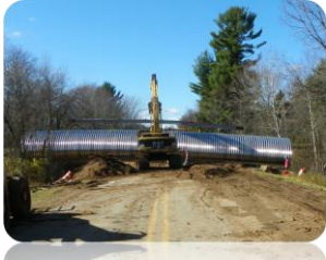
The above photo shows the assembled 13,000 pound culvert being lifted and ready for installation at the Bark Creek crossing of State Road.
