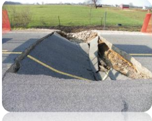
The above picture is a portion of Barry Street in Blendon Township that was damaged from the April storms.
