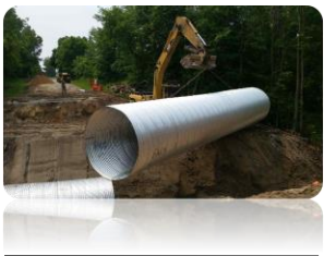
The above photo shows Road Commission crews replacing a culvert on 104 th Avenue in Crockery Township.
