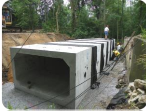
The picture above shows a box culvert installation along Leonard Street in Polkton Township.
